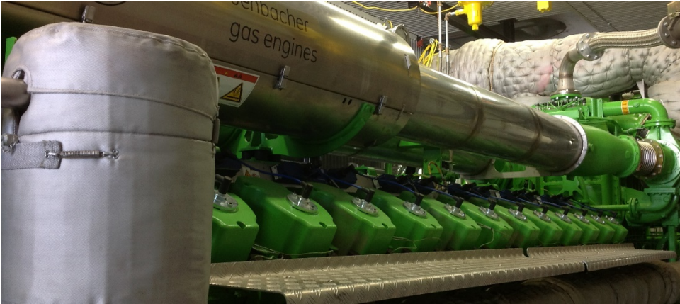
Pic 1: Cogeneration Engine Installation
