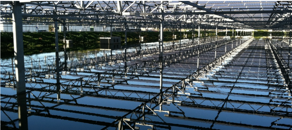
Pic 1: 4 acre water retention pond beneath solar field
