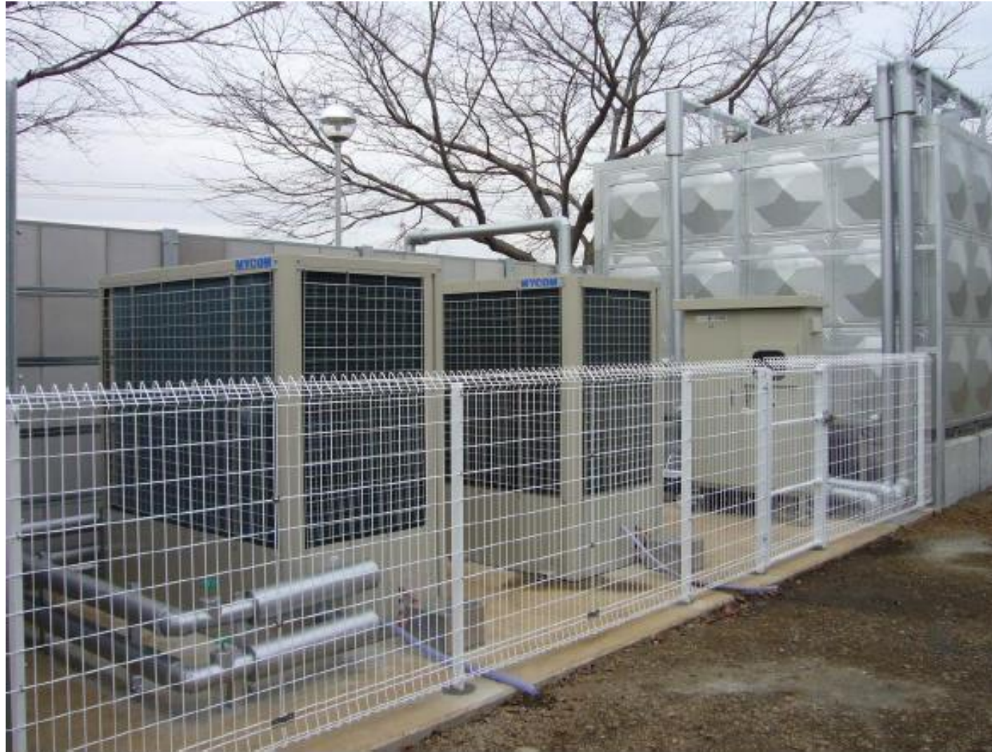
Mayekawa (MYCOM) 22.5-ton air-source system
