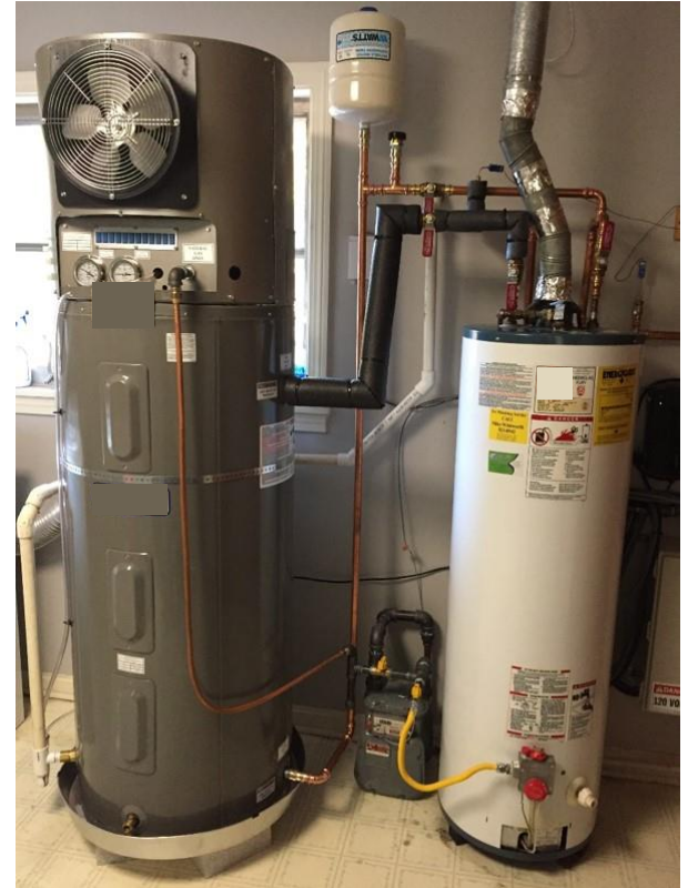
Gas HPWH operating at field site in 2017
