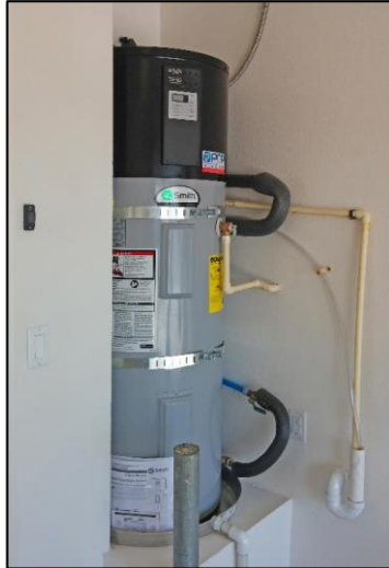
Electric Heating and Water Heating
